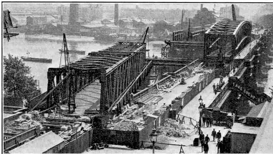
The Centre Span lying on the Bridge, ready to be rolled into its final position
