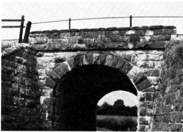
A 19th century stone arch bridge, carrying a railway line: this technique has remained unchanged after 2,000 years.
