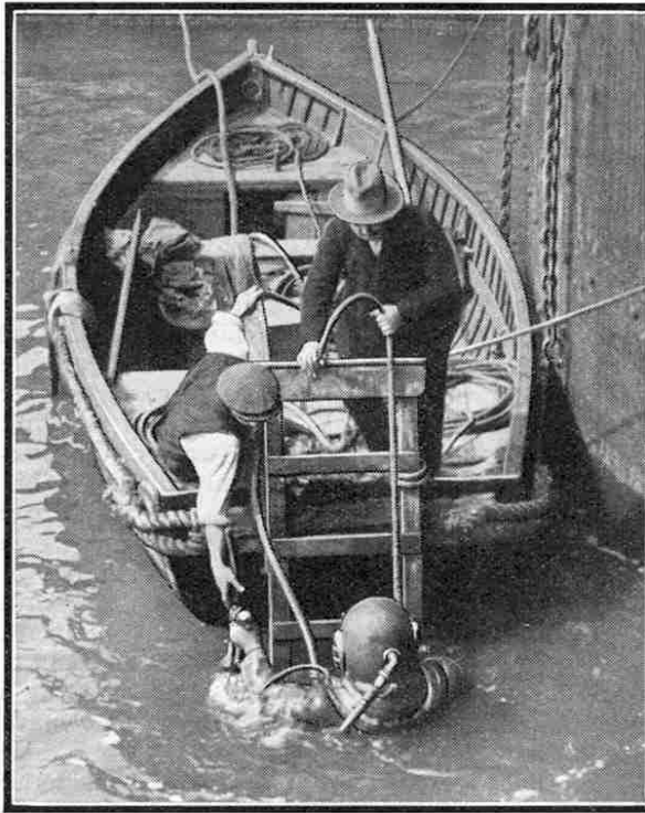
A diver at work in the Mersey, where he is caulking a leak in the gate of the Langton Graving Dock. Photograph by G. A. Collins, Liverpool.
